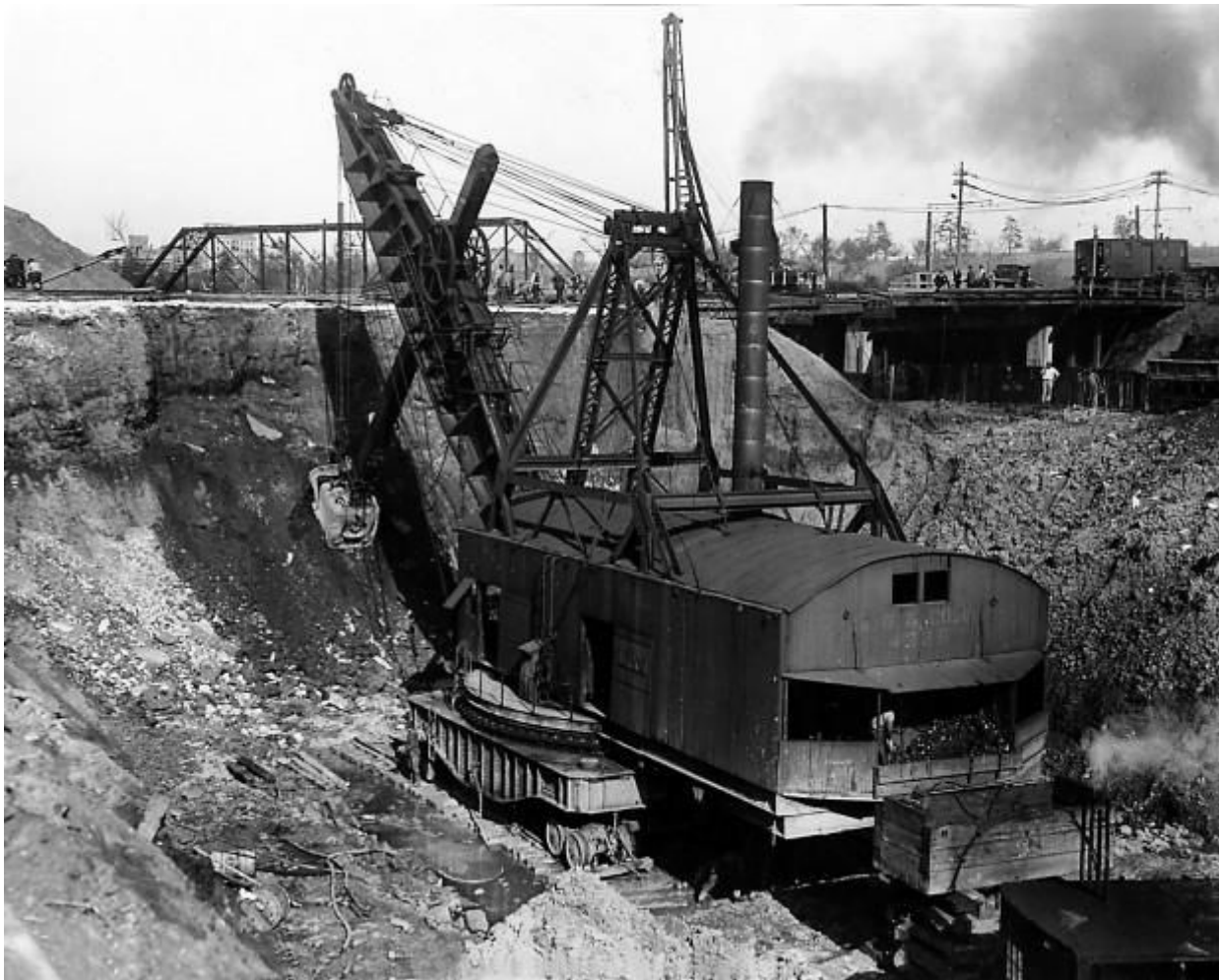
Creating new tunnel for River Des Peres south of Oakland/ Forest Park
